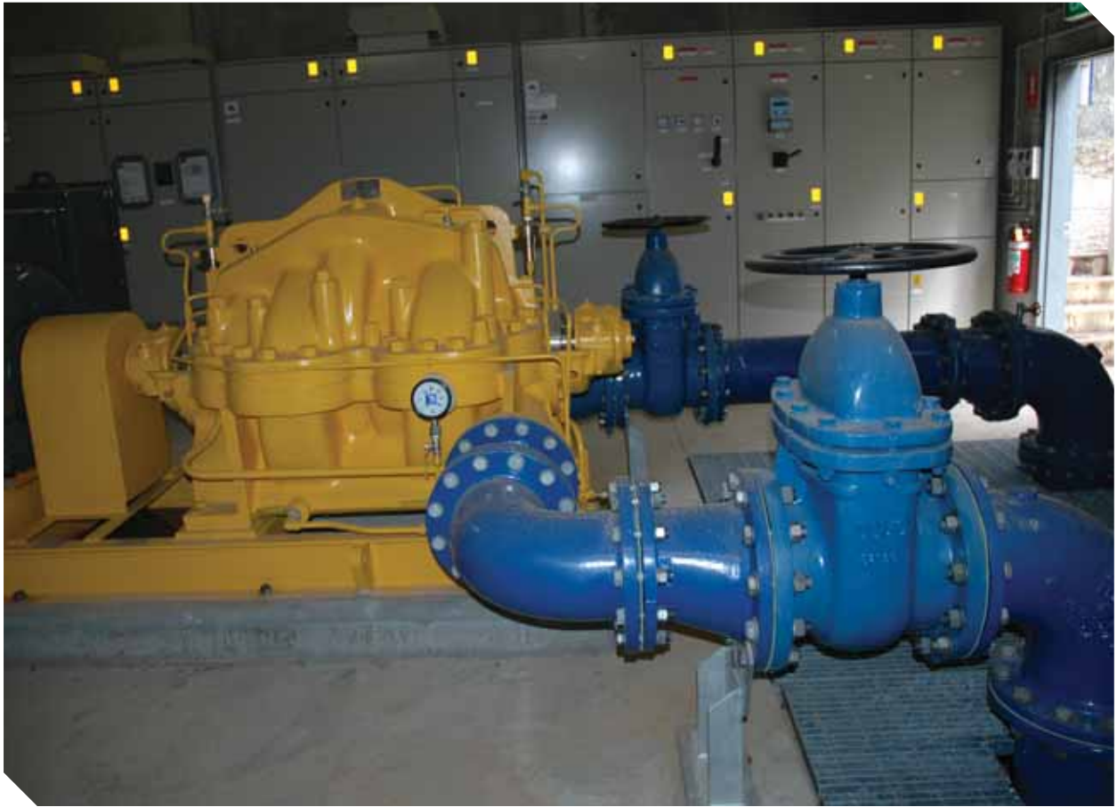
Sunday Creek pump station
