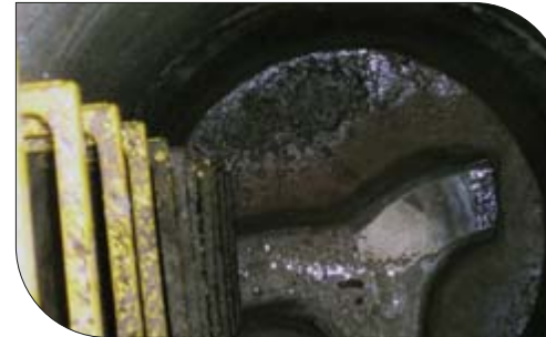
Blockage in Authority's sewer main
