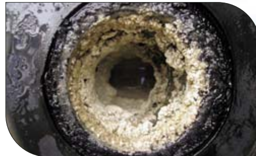
Blockages in property drains
