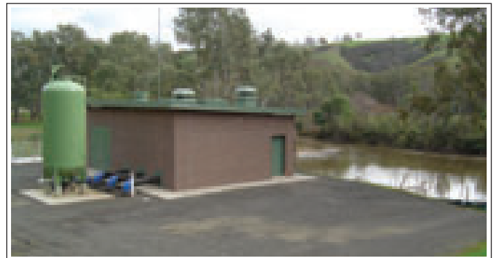
Picture Pump Station on the Goulburn River at Tallarook.
