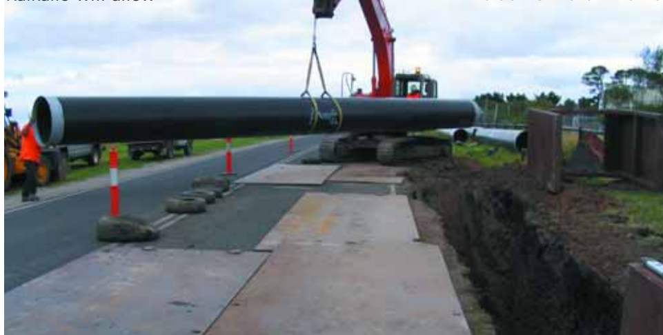
Construction of the 22km water supply pipeline from Mt. Ridley to Wallan
