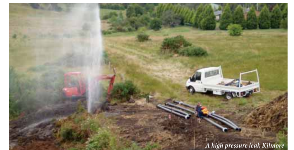
A high pressure leak Kilmore
