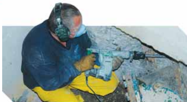
Mick Meeny replacing a section of cracked pipe at the Seymour pump station
