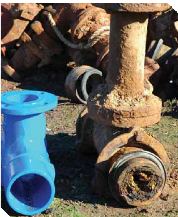
A corroded unlined cast iron fitting from Girgarre, beside a new fitting
